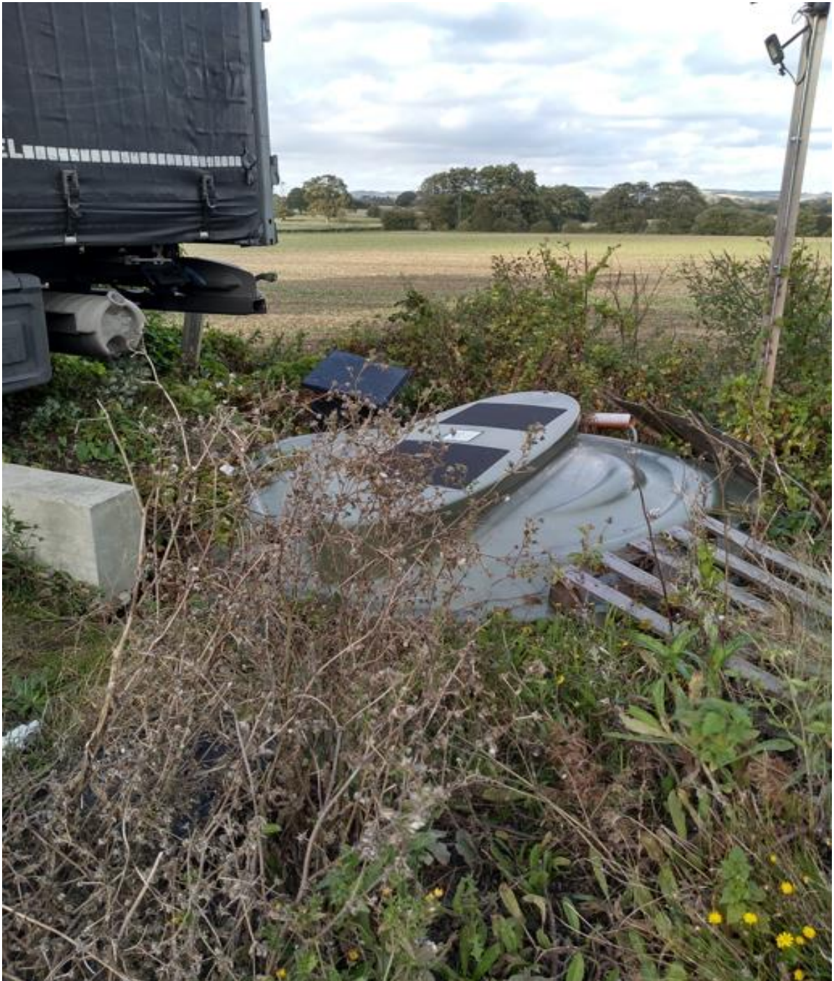
Figure 9 – waste water treatment system
