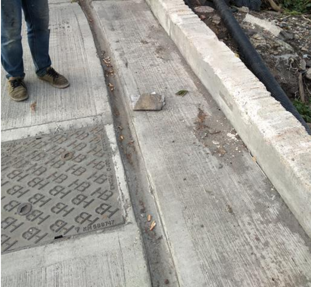
Figure 10 – kerbing, trough drain and interceptor cover.
